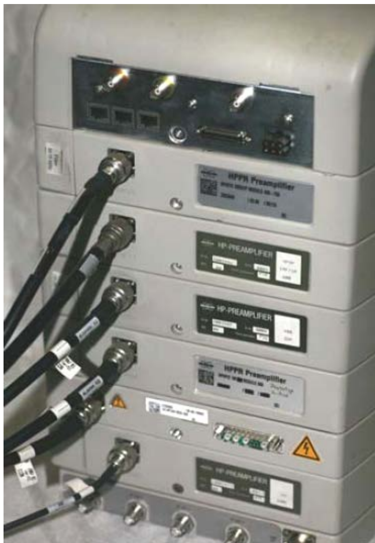
Figure 3.2: Transmitter Cables (only) Wired to Back of the Preamp
